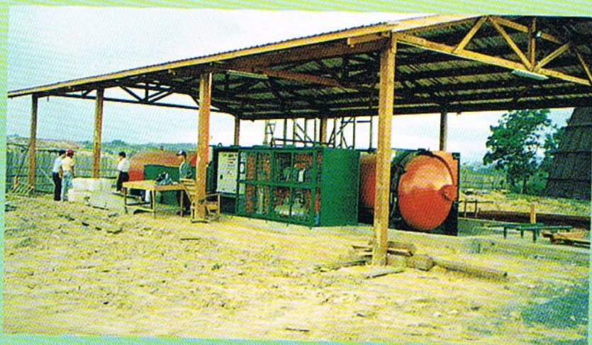
Newly Installed DWT T10 impregnation plant
