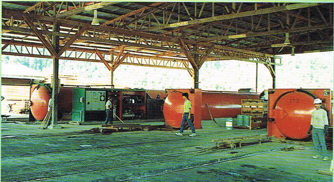
3 units DWT T10 impregnation plants installed in Sabah, Malaysia.
