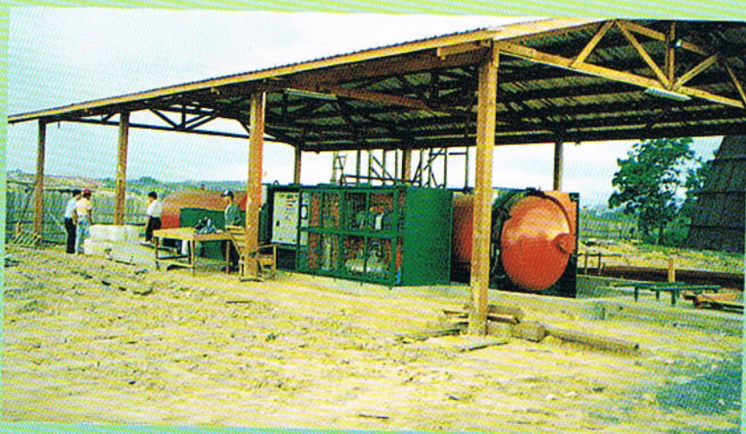
Newly Installed DWT T10 impregnation plant
