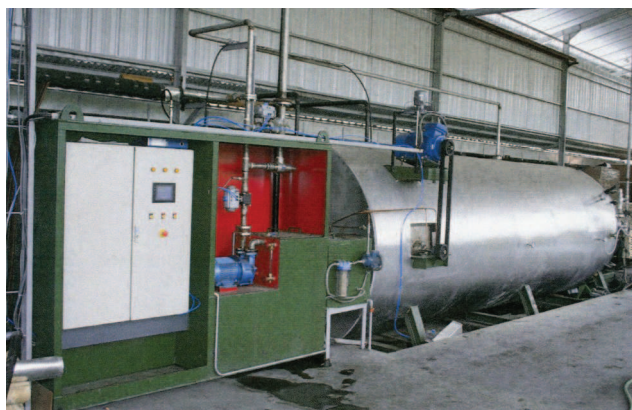
The entire plant fits easily into existing production facilities
